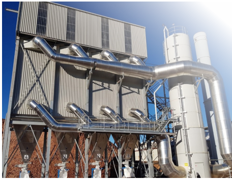
Flue gas heat exchanger
