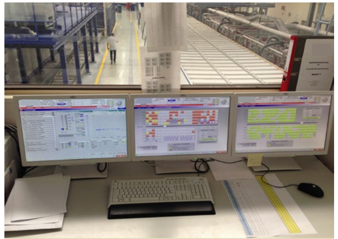
Trocknerleitsystem Dryer control system
