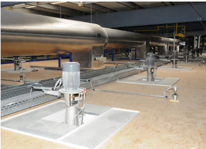
有旋转风机的干燥机屋顶 Dryer roof with rotary fans
